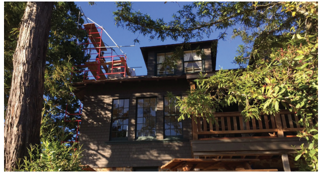
Boston Brick & Stone's 35-foot scaffold looms over the Inn as masons restore and improve airflow in the 112-year old chimney.
