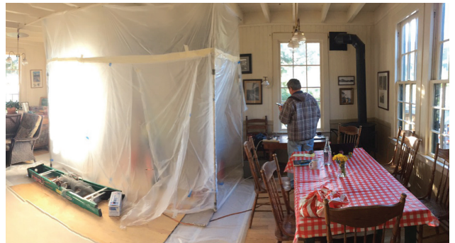
Boston Brick & Stone plastic barrier helped keep the Inn clean. During "demo" (demolition) a fan was atop the chimney sucking dust and dirt out.
