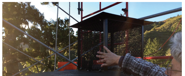
The new spark arrestor they created for the top of the parlor chimney.
