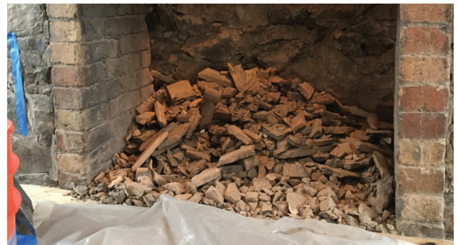
Remnants of the 112-year old clay chimney liner await removal from the parlor fireplace. Note the missing firebrick at the back. We're deepening the "firebox" as part of improving the "drafting" of the fireplace. Historically correct firebrick, the same kind of brick used originally, will cover the back wall and look no different than the fireplace we remember after a few fires.
